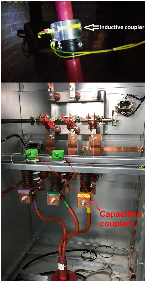
Figure 2: Tested wired medium in an underground mine shaft.
